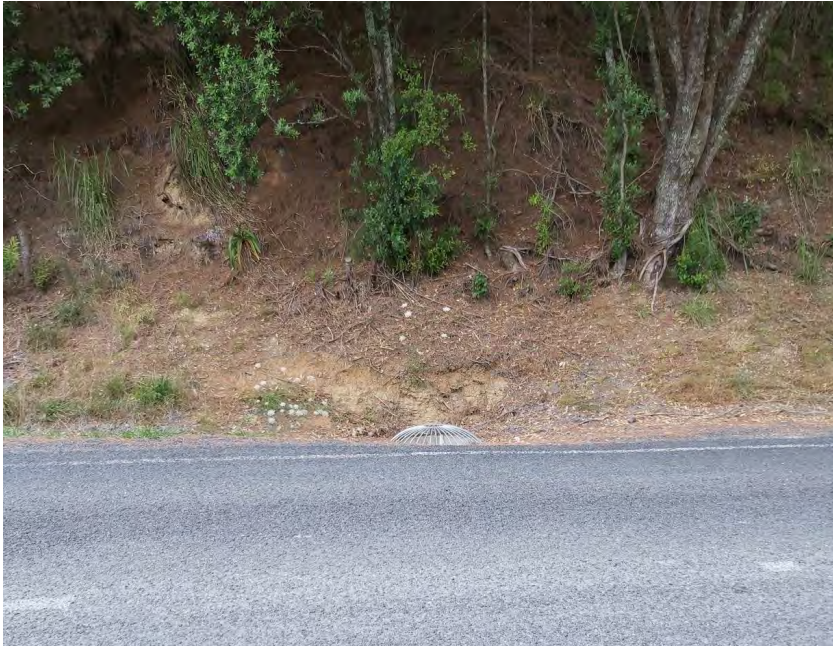
Photo 8: Culvert running under Mahurangi East Road & forming a point source discharge across the proposed track above site # 17. The culvert is the opposite side of the road to the reserve.
