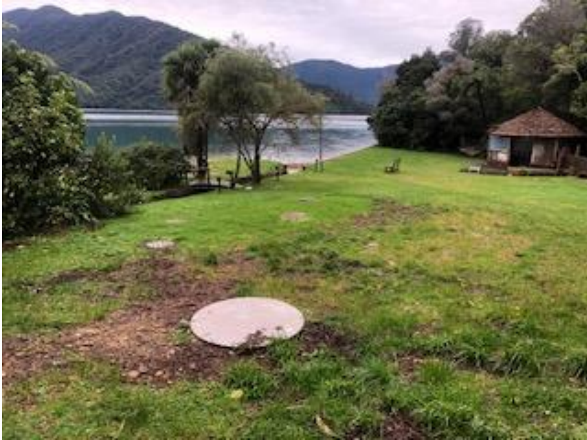
ANC5 - Primary WW Tanks
