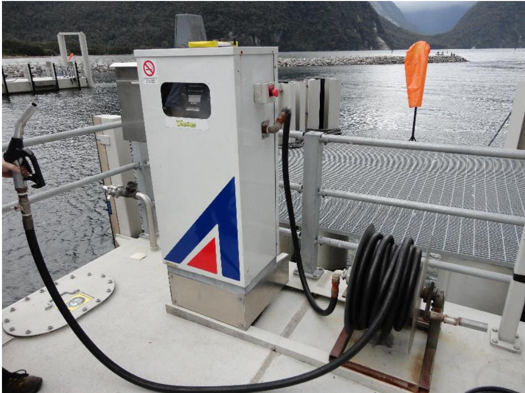
Photograph 3: Photo showing one of the dispensers located at the end of the pontoons
