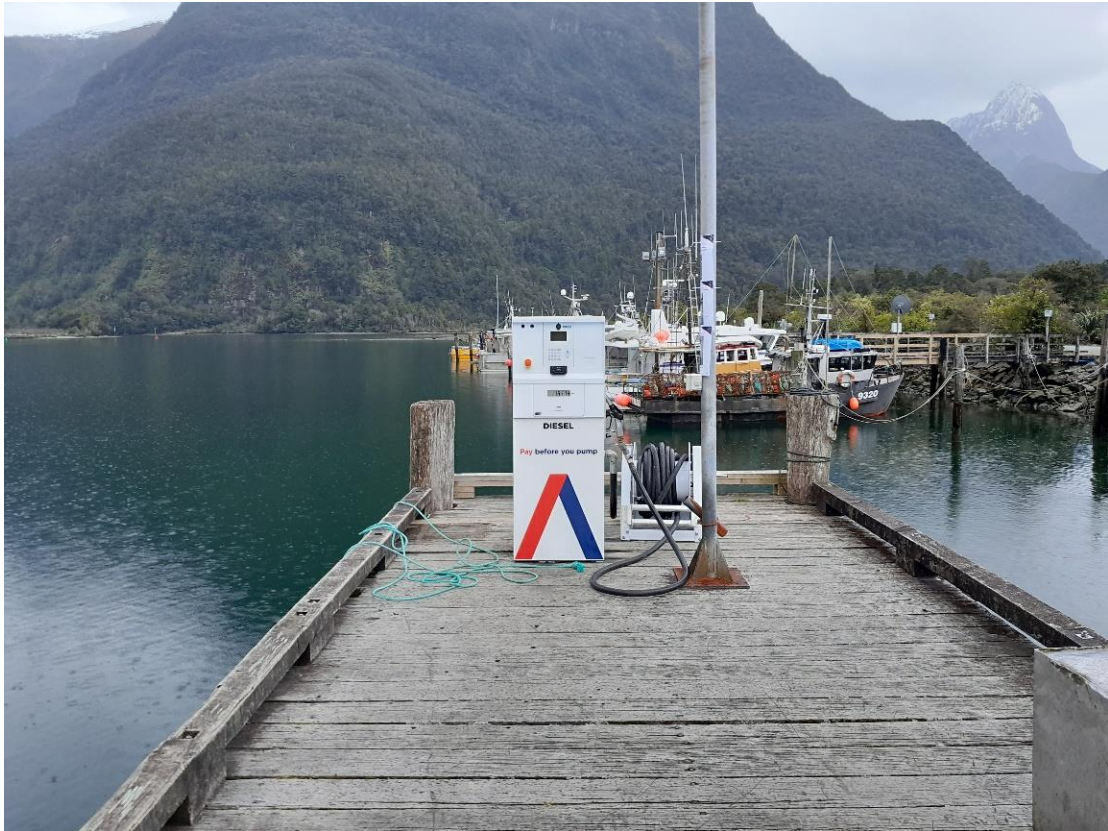
Photograph 5: Photo of the dispenser at the end of the wharf
