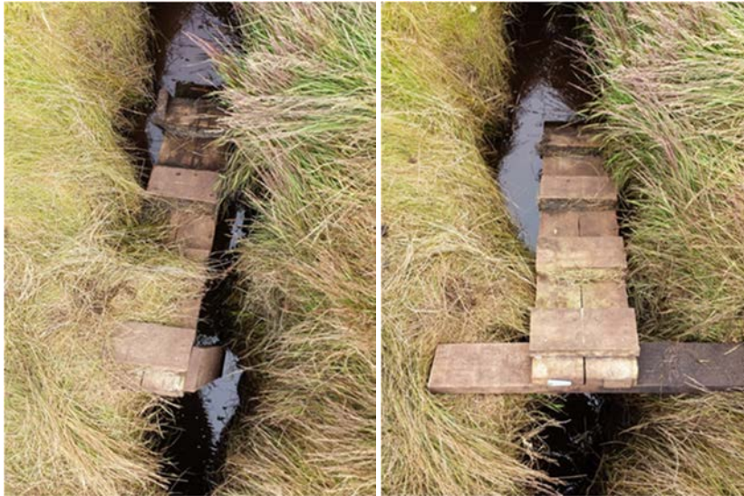
Figure A9.4 Ramp P913 at Sandy Bay, Enderby Island before alteration (left panel) and following alteration (right panel)
