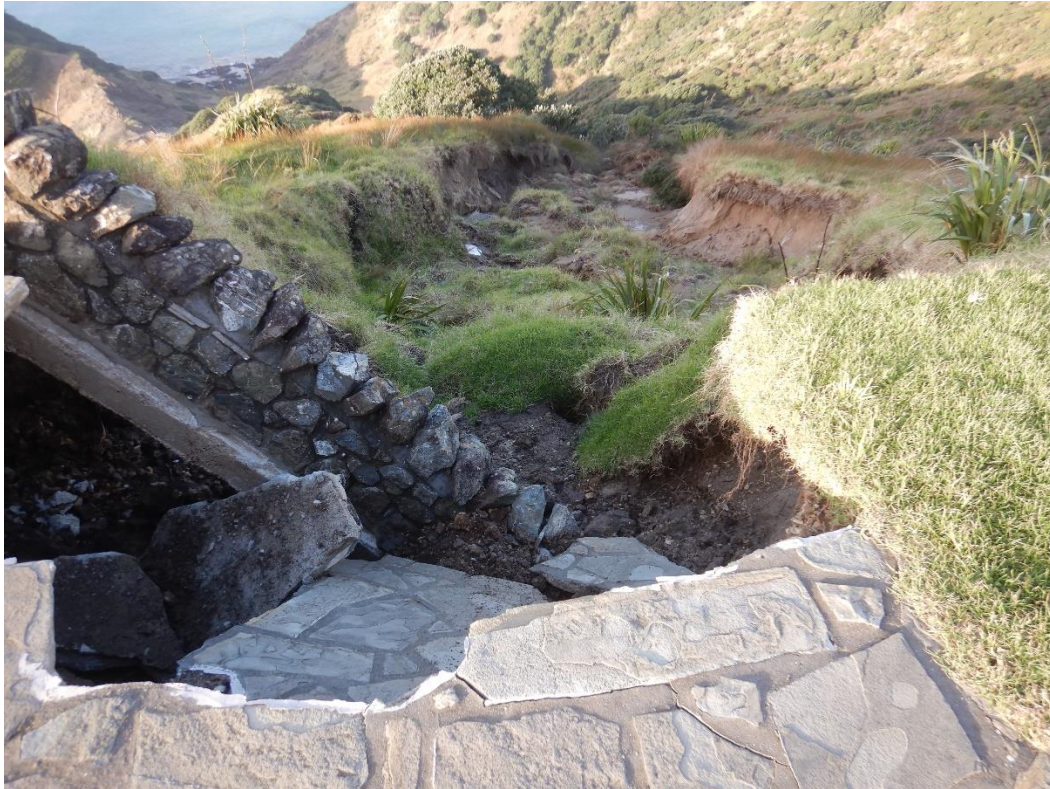
Figure 12: A significant amount of soil material has flowed down the steep slip path from under the collapsed wall and paving area.
