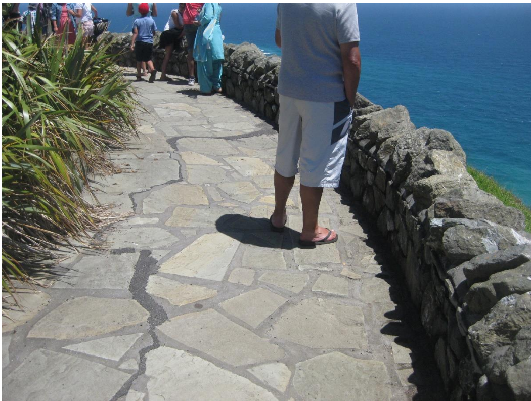
Figure 10: Evidence of cracking and settlement of the paving over the filled area after repairs had been undertaken in late 2013.
