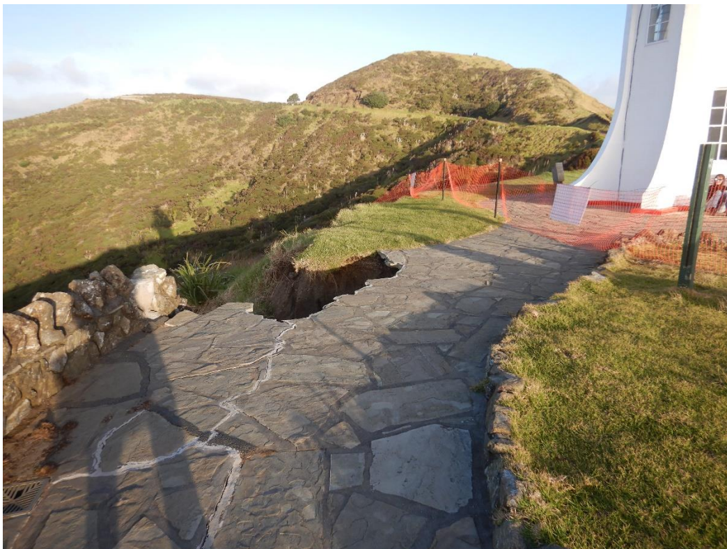
Figure 11: Failed section of paving and wall on the eastern side of the lighthouse area.
