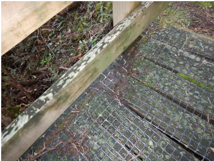
Figure 2: Deck mesh lifting on bridge 023974
