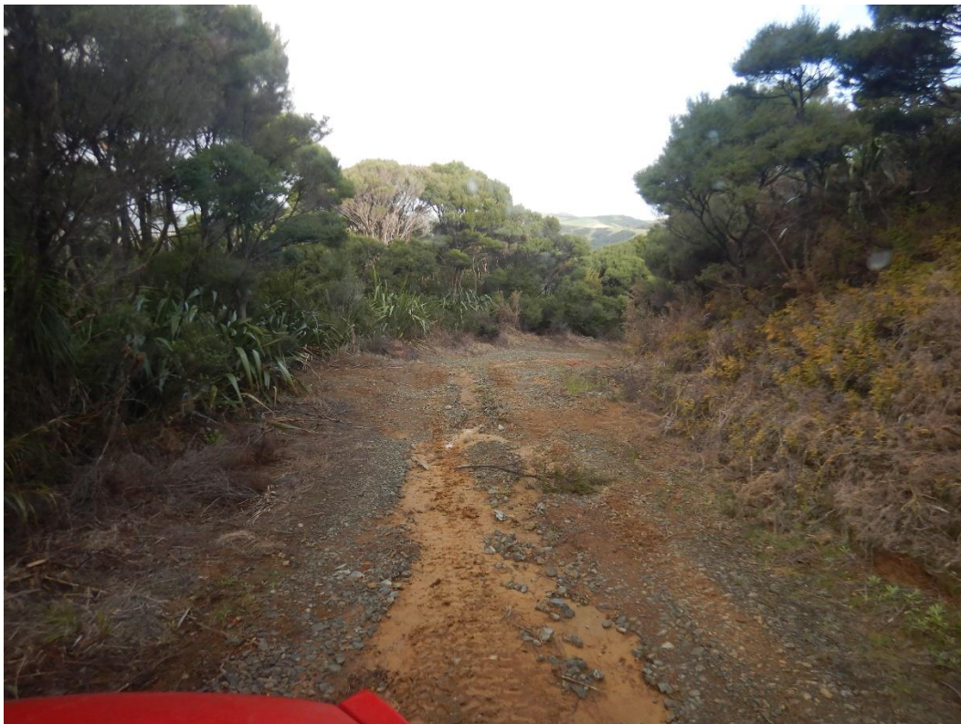
Figure 6: Blocked cut-outs result in water flowing some distance down the road causing extreme erosion.
