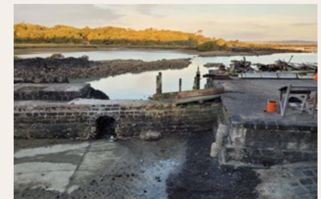
Photo during restoration works of the Rangitoto tidal swimming pool, with A-frame shed and decking removed, January 2024. Photo: DOC
