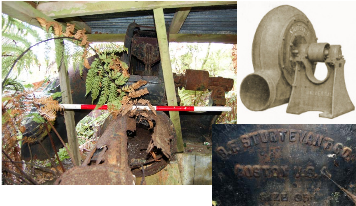
Figure 5: cast iron Sturtevant fan under rough corrugated iron roof. “Monogram” model, manufactured in the 1920s – 1940s. A large volume fan, adapted for exhausting smoke fumes and gasses from engine-rooms, laboratories and kitchens (see B. F. Sturtevant, n.d., and also www.sturtevantfan.com ).
