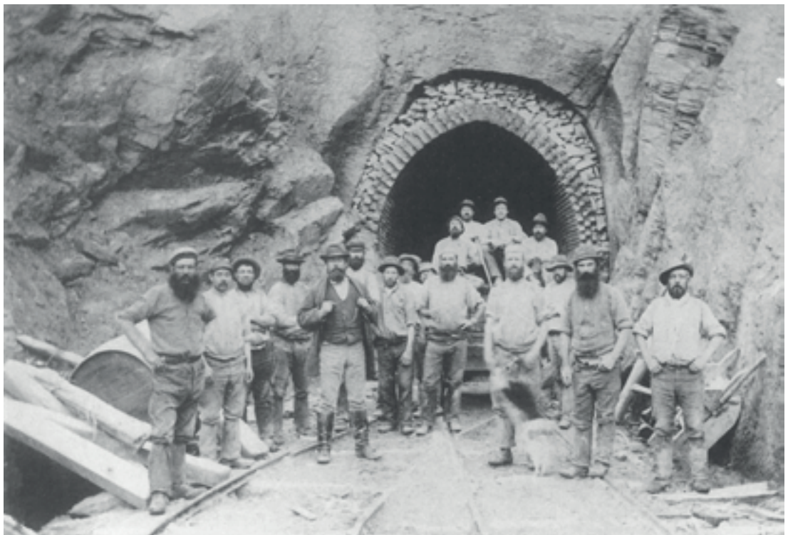
Figure 7. Tunnel techniques. A great image from c. 1895 showing 18 men working on tunnel construction. Tunnel portals like this were typically brick-lined for stability. If the rock deeper inside was unstable, they were lined throughout. An arched wooden formwork (not seen here) was used to form the bricks into a curve and hold them in place until the mortar set and they became interlocked. The formwork was then progressively moved along. As seen here, stones were then stacked on top of the brick lining to fill in the void between the bricks and the rock face. Bricks for these Otago Central Railway tunnels were made at Outram and transporting them to the remote tunnel sites was a logistical challenge that may have involved boats and pack horses. This is the 122-metre-long Duck Point Tunnel #4 near Parera in the Taieri Gorge. The chap with the waistcoat is possibly one of the Gore brothers (contractors). Photo: F.A. Coxhead, courtesy of Hocken Library.
