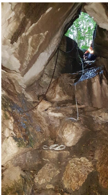
Figure 2 Existing access down into the Moria Gate. Chain 'hand rail' at left threaded through eyelets. Photo provided by client.
