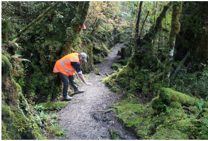
Figure 7 Ōpārara track; Upgrades here include raising the track surface by 200mm and retaining the edges with limestone rocks in gaps where there is no existing bedrock. Photograph by J.Head 6 August 2020
