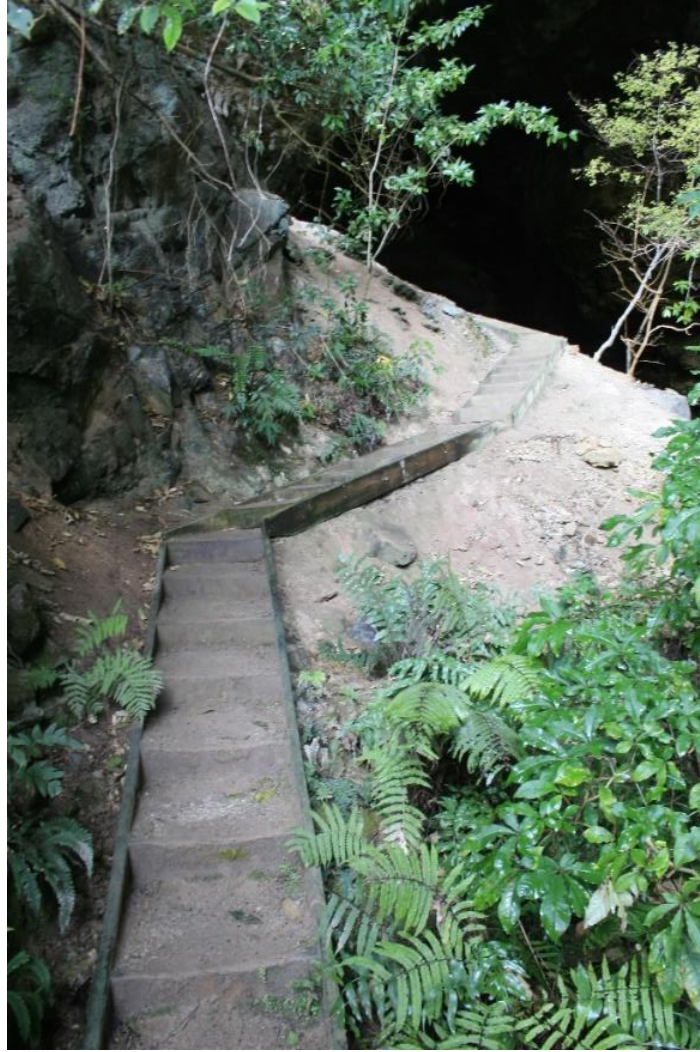
Figure 16 (previous page) Ōpārara track; Difficult section of timber stairs passing under possibly hazardous area (potential for rockfall). This section of track will be retired, and the stairs removed. An alternative safe more accessible access to the arch entrance is proposed. Photograph by J.Head 6 August 2020.
